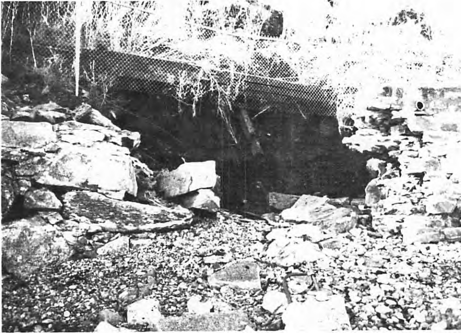
Washed out walkway between Sheep Point and Rough Point.
