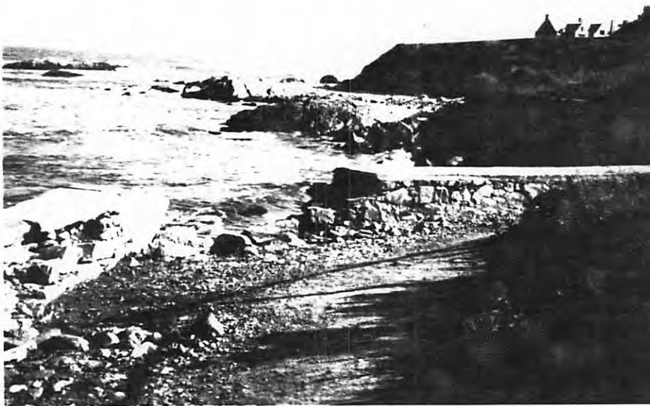
Washed out seawall between Sheep Point and Rough Point.
